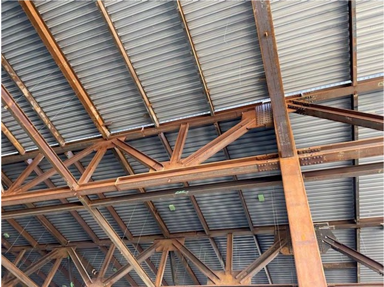
Looking up at the primary/secondary truss configuration from the exhibition level, image courtesy of RJC Engineers
