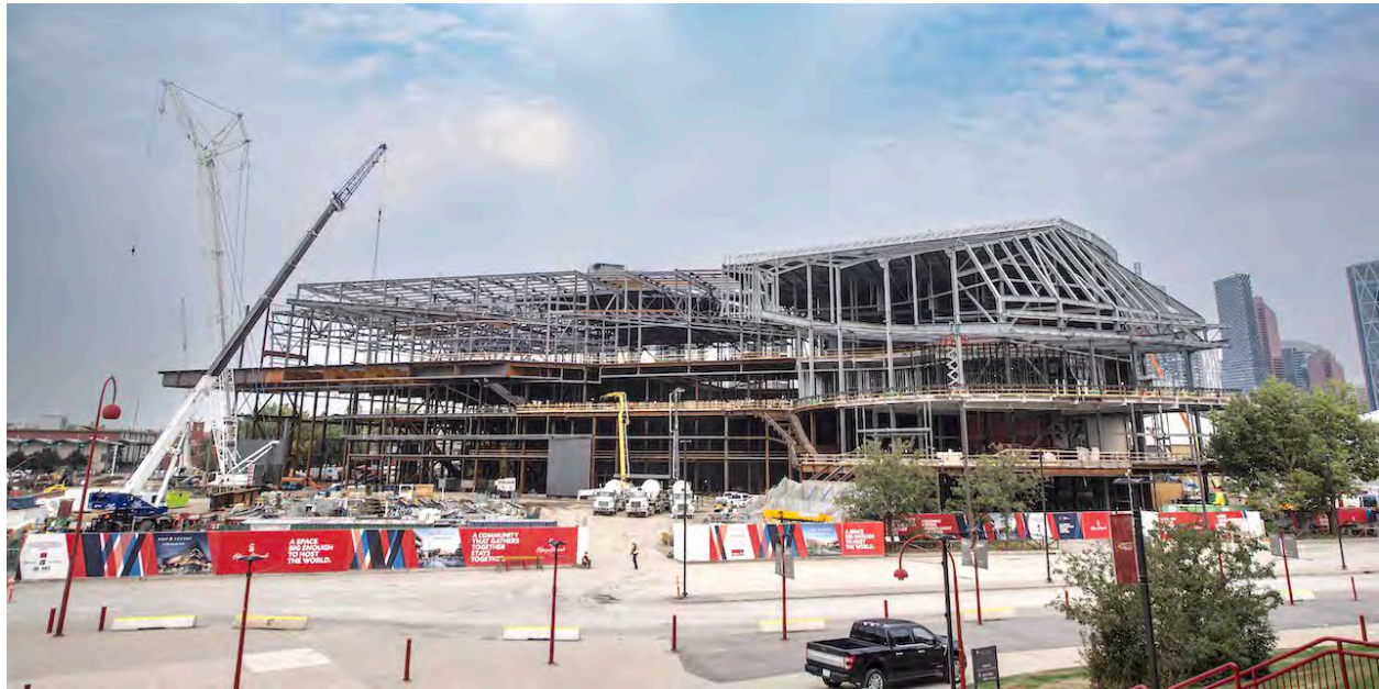
Looking northwest to the building’s steel frame, image courtesy of CMLC and Calgary Stampede
