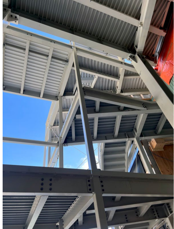
RJC ENGINEERS — View of the structural steel framing that makes up the new atrium entryway and stairs.
