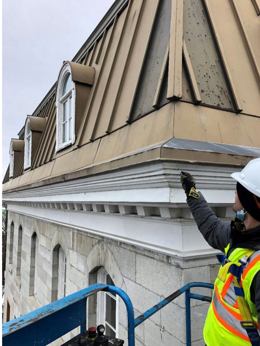
PHOTO COURTESY RJC ENGINEERS – Pictured is RJC Engineers completing a detailed condition assessment of the building envelope and masonry structure.
