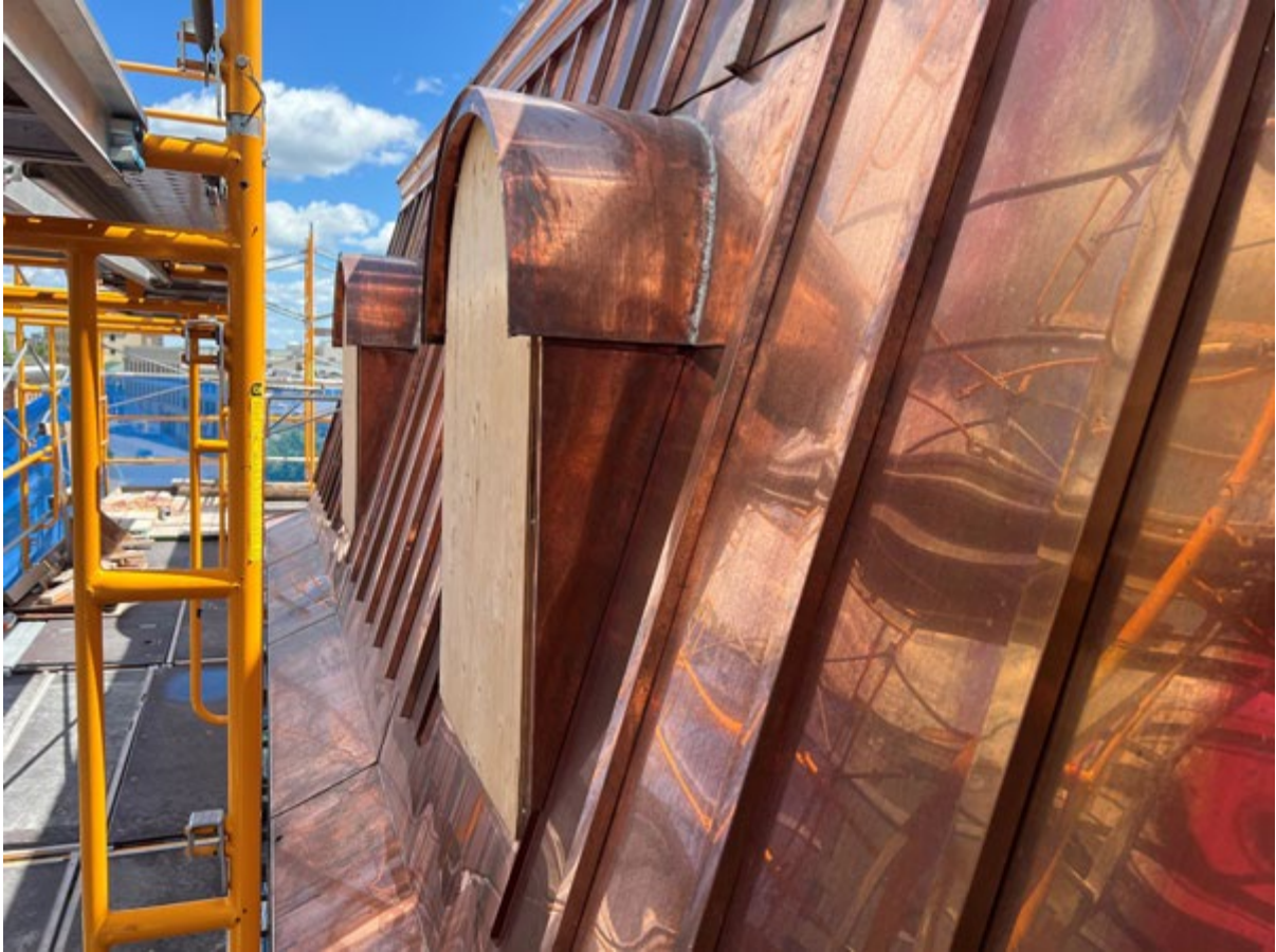
PHOTO COURTESY RJC ENGINEERS – As part of restoration a new copper mansard roof was installed.
