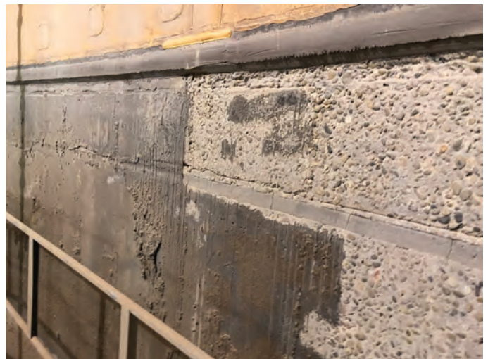
Fig. 3: Partially removed pre-existing coal tar coating
