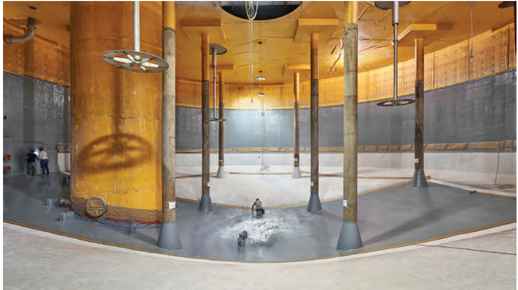
Wastewater Treatment Plant: Gold Bar Digester No. 3
